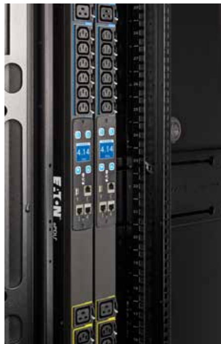
Figure 1. Rack PDUs with racks from the same vendor ensure compatibility, which enables agility in the data center.
