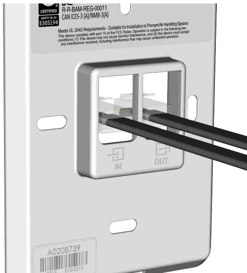
Figure 3. Insert Ethernet Cables
